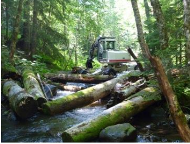
Restoration efforts like this large wood placement project enhance stream function and improve habitat for salmon, steelhead, and resident fish.
